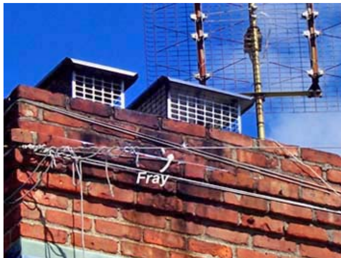
It's the time of year to check your antennas and supports. Here is a recently-discovered frayed rope, barely clinging on to Karl's chimney.
